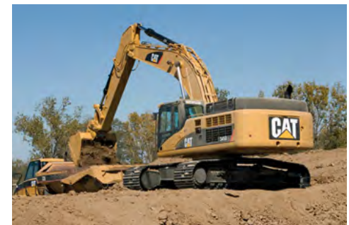
Figure 4.4.3.3 - Crane mats will be placed by a CAT Track 380 Excavator to establish a stable boring platform
