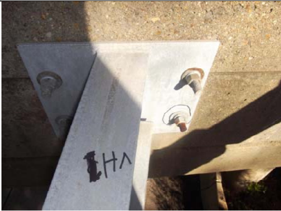
Failed mounting bolt (circled)
