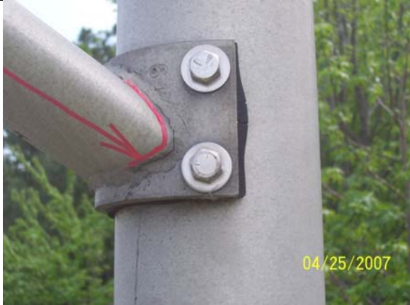
Lower arm of luminaire chord has a 3.5" fatigue crack in weld at connection to pole
