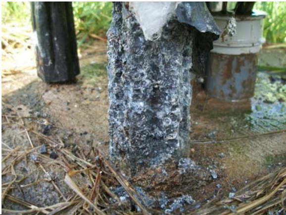
Corrosion with 1/8" deep pitting on breakaway couplers
