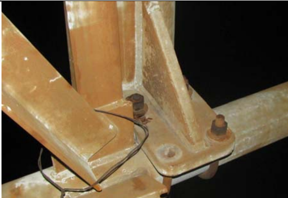
U-bolt sheared at left front pole to bottom chord Connection
