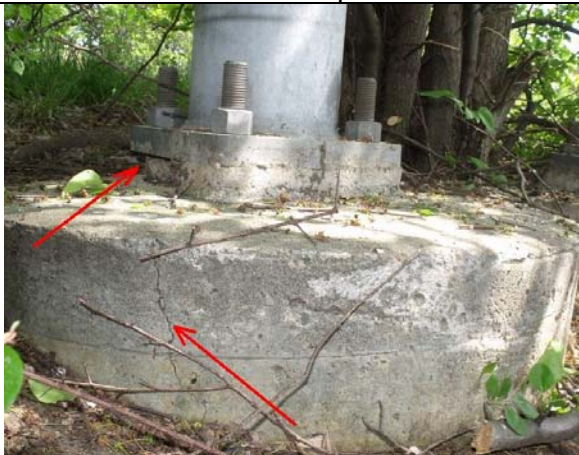
Deteriorated grout pad and cracked pedestal
