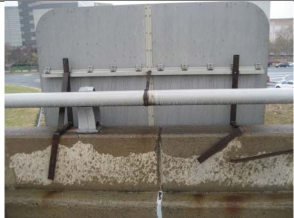
Twisted anchor clamp over the parapet
