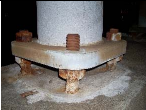
Rusted anchor bolts and missing nut
