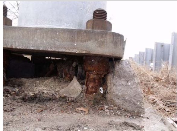
Severely corroded anchor bolts exposed when grout has fallen away
