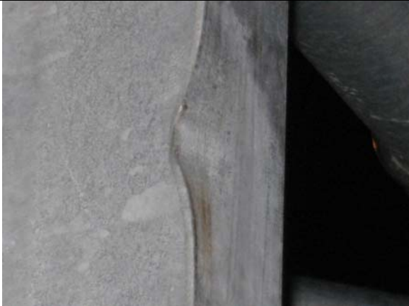
Damaged & bent flange of vertical hanger
