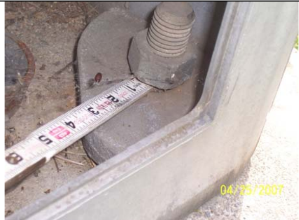
Loose anchor bolt nut at luminaire base
