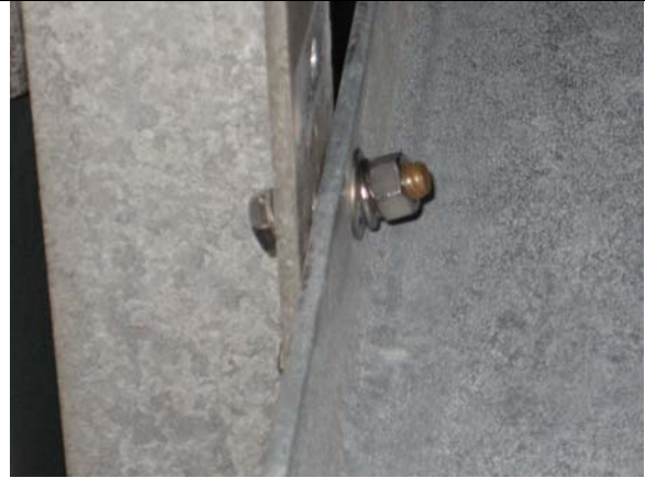
Poor vertical hanger connection with the Z-bar
