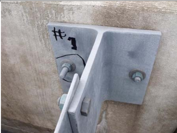
Failed bolt (circled) at parapet mount.
