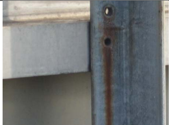
Missing bolt at wind beam to vertical hanger connection
