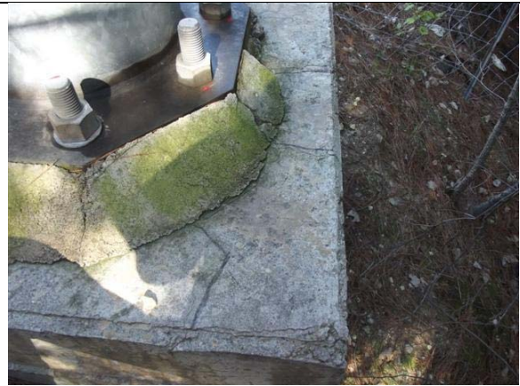
Deteriorated and cracked grout
