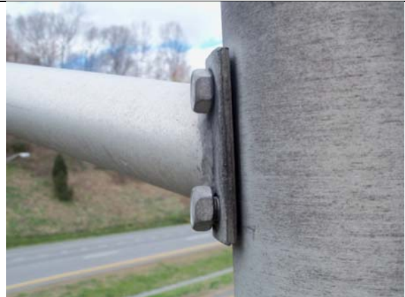
Two of four bolts loose in top chord connection to luminaire pole
