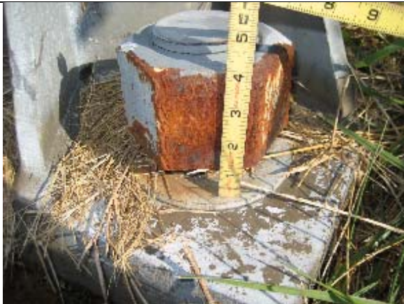
Loose anchor bolt with 1" gap between nut and base plate
