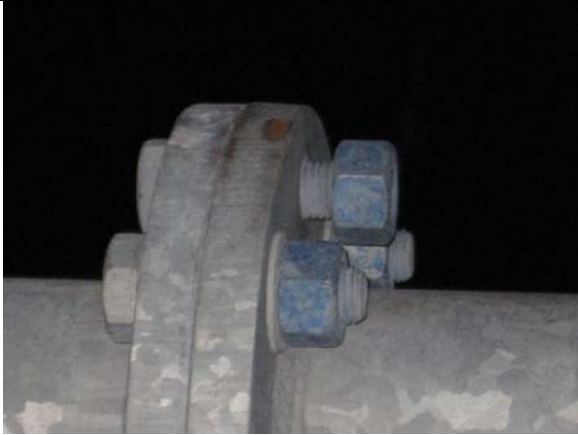
Loose Bolt at splice plate.
