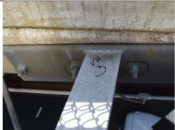
Two failed bolts (circled) at parapet mount
