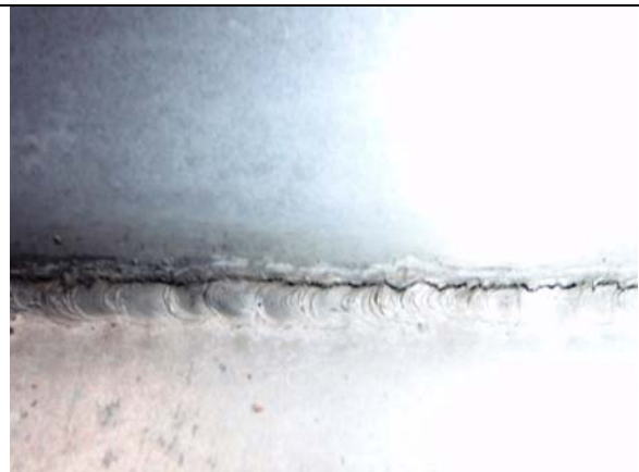
Crack in luminaire bracket saddle to connection plate weld
