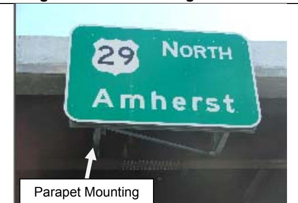
Figure 4 – Parapet Mount Sign Structure (Note that “Parapet-Mount” sign structures may also be attached to bridge girders in addition to bridge parapets)
