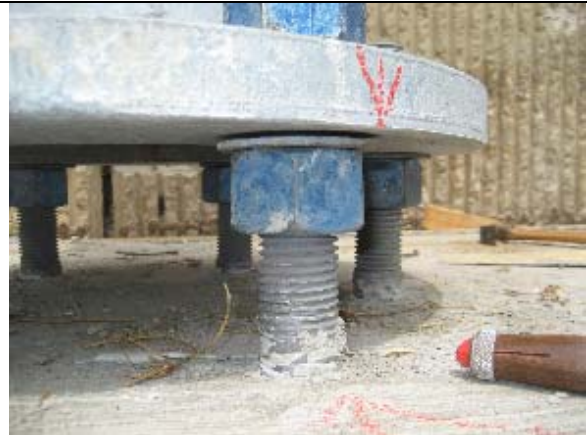
Leveling nut is loose and gap is too high
