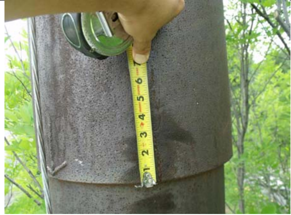
4" vertical crack at the slip joint
