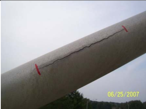
6" crack in lower chord of luminaire
