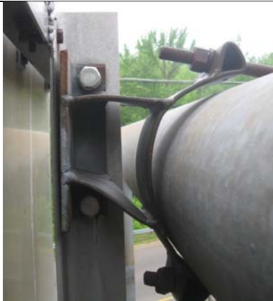
1 1/2" gap between upper chord and connection strap
