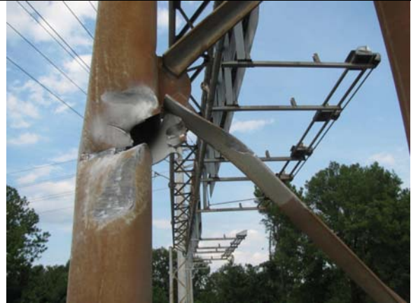
Column torn and bent 3" at point of impact
