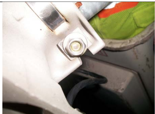
Nut on strap bolt for signal from pole lacks 50% thread contact
